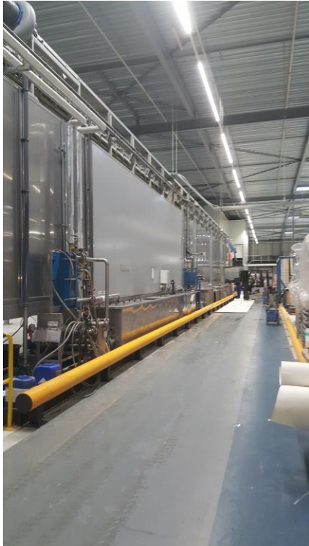
Image 3 Circulation system with fixed pipes and baths
